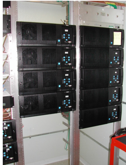
FIGURE 1 Kitsap VHF Base Station Equipment
